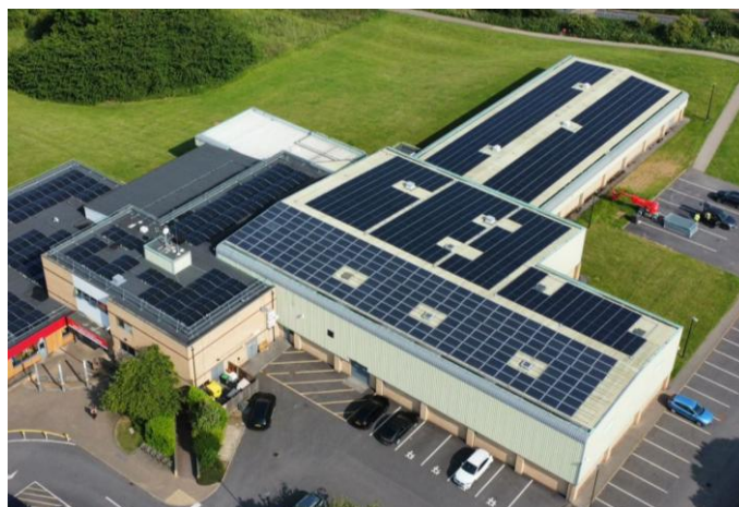
Solar panels on West Lindsey Leisure Centre (Gainsborough), July 2025
